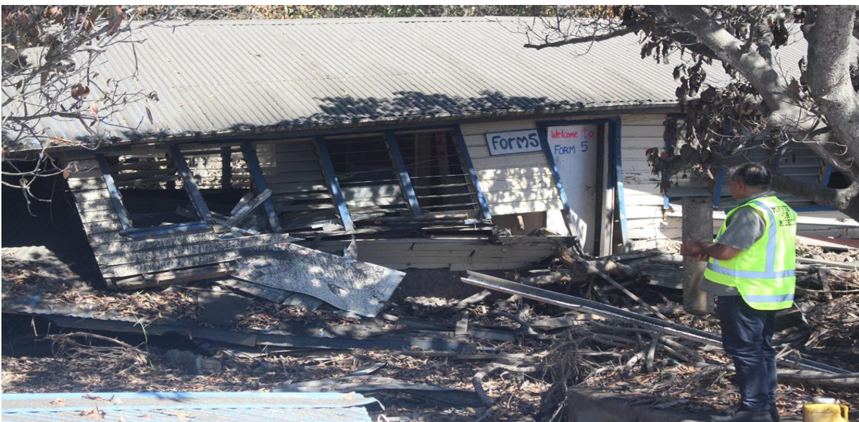
Pic: Hon Deputy Prime Minister and Minister for MEIDECC looking at damages to Tupoto'a College (Source: MEIDECC)
